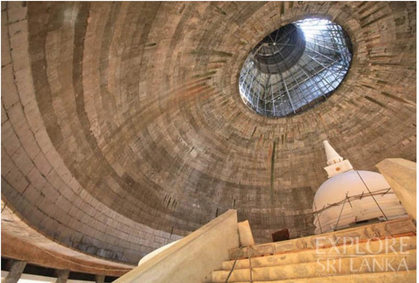
Inner Stupa of the Mahaweli Maha Seya in its final phase of construction
